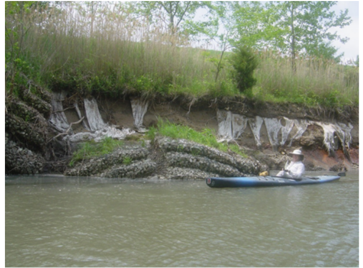
Structural controls designed to protect the ash ponds from the river have failed.
